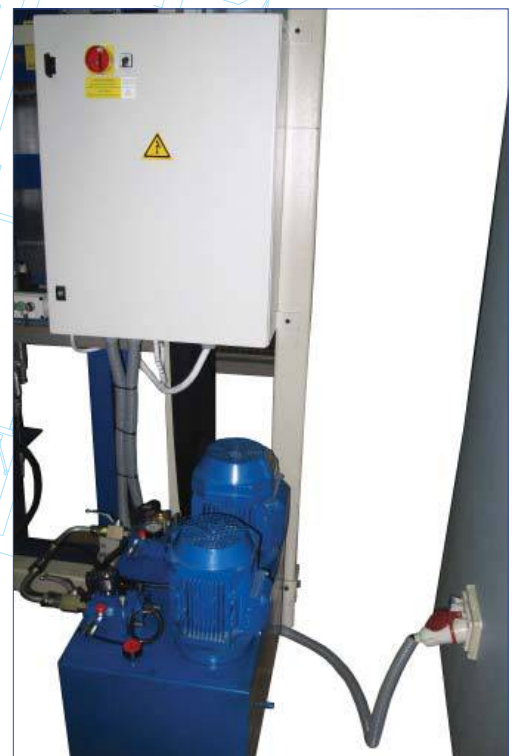
Figure 20. Electrical control panel.
