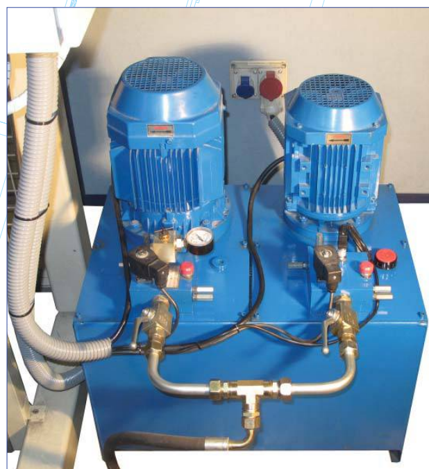
Figure 17. Central Hydraulic Unit.
